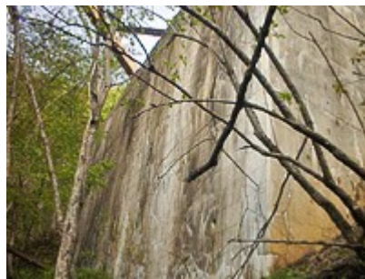
ひび割れ補修前
